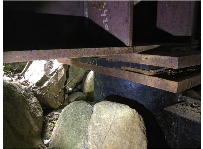
Typical Bulging of Bearings
