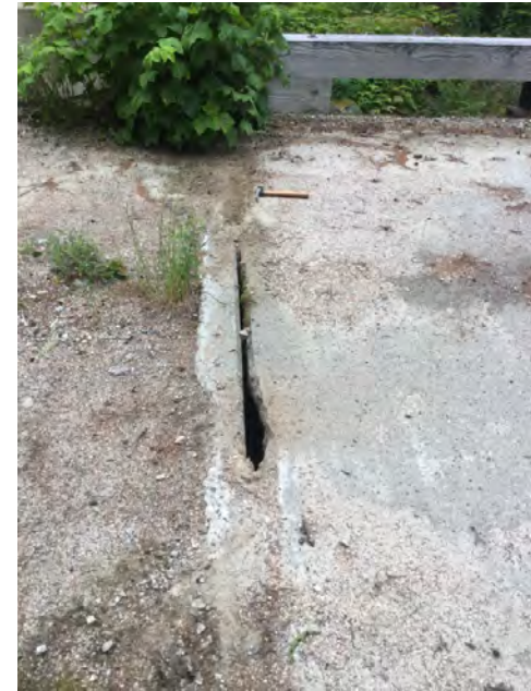
Left Abutment Damage to Ballast Wall and Deck Panel
