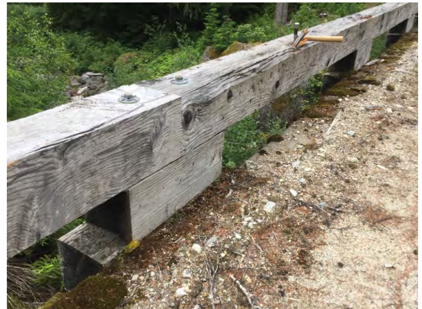
Rotten Guardrail And Blocking
