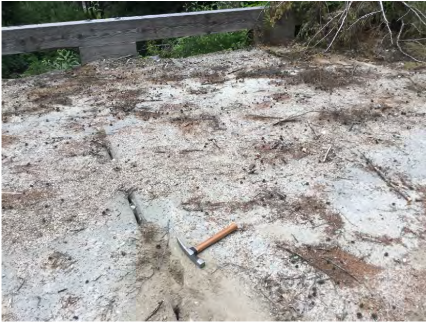
Damage to Right End Deck Panel & Typical Missing Sealant/Compression Seal
