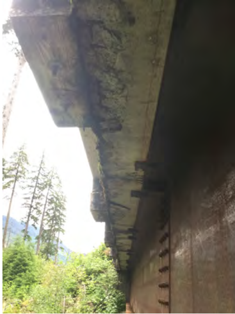
Typical Spalling of Downstream Guardrail Anchorage
